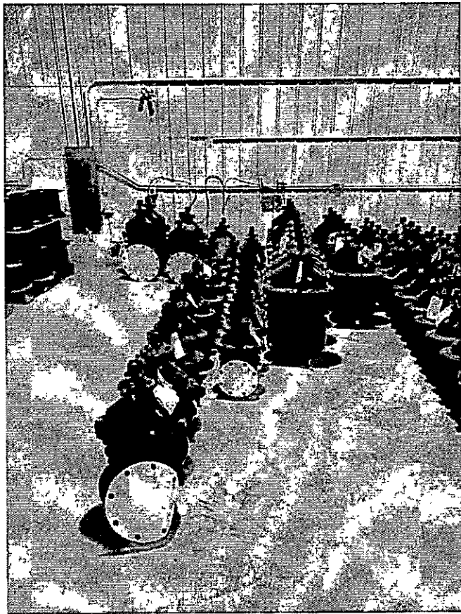
PICTURE 1 - GATE VALVES ON SITE
